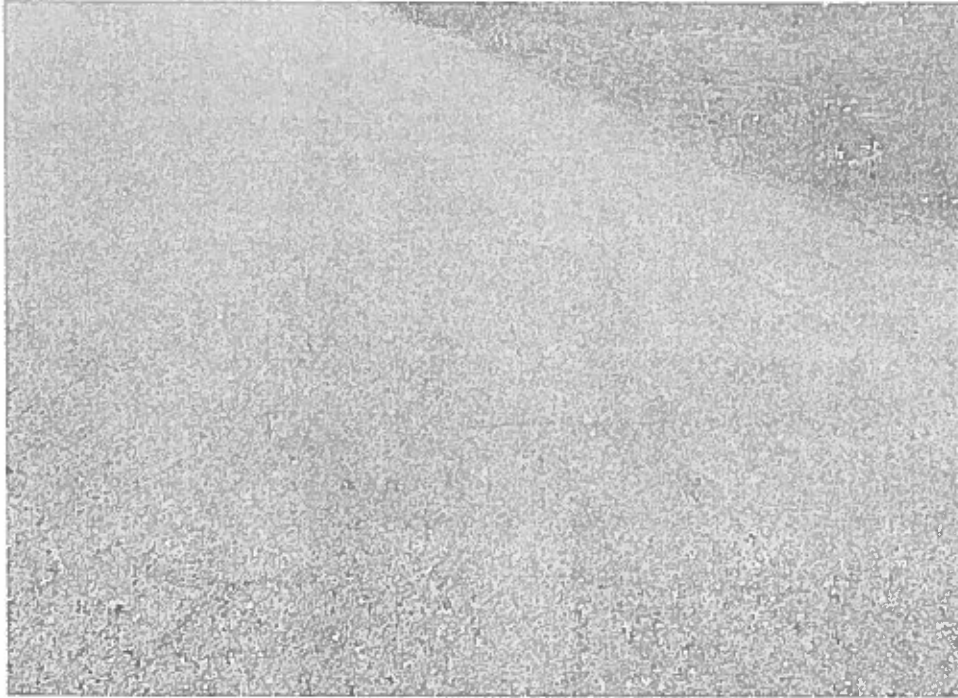
Figure 1: Light cracking and light raveling
