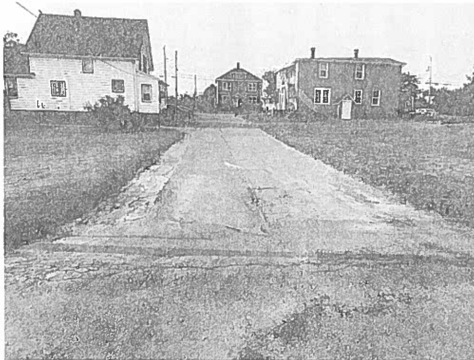
Figure 6: Church St - Insufficient storm pipe cover, cross slope, and drainage - Recommend further investigation.
